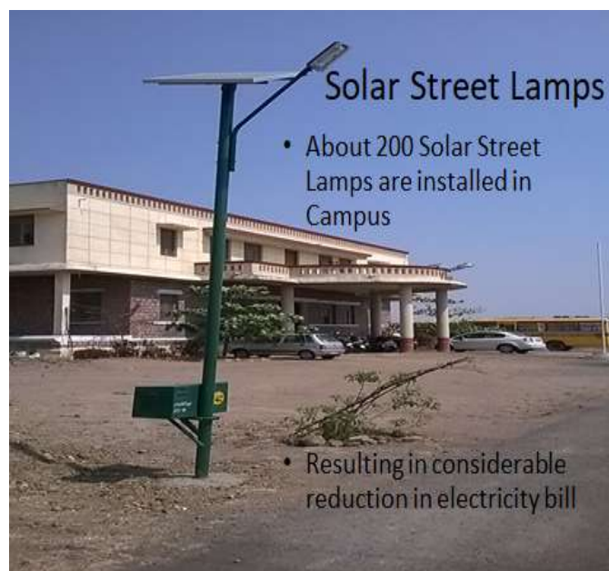
Plate 2: Solar Powered Street Lamps
