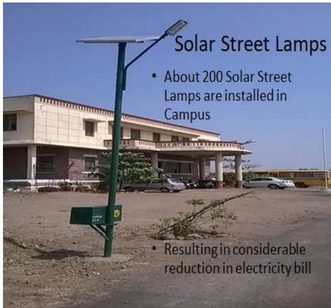
Plate 2: Solar Powered Street Lamps
