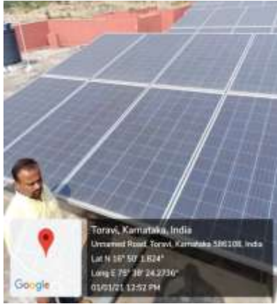
a) Roof Top Solar Panel
