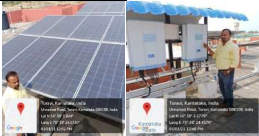
a) Roof Top Grid Connected Solar Panel
