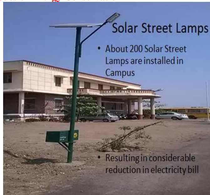
Plate 2: Solar Powered Street Lamps
