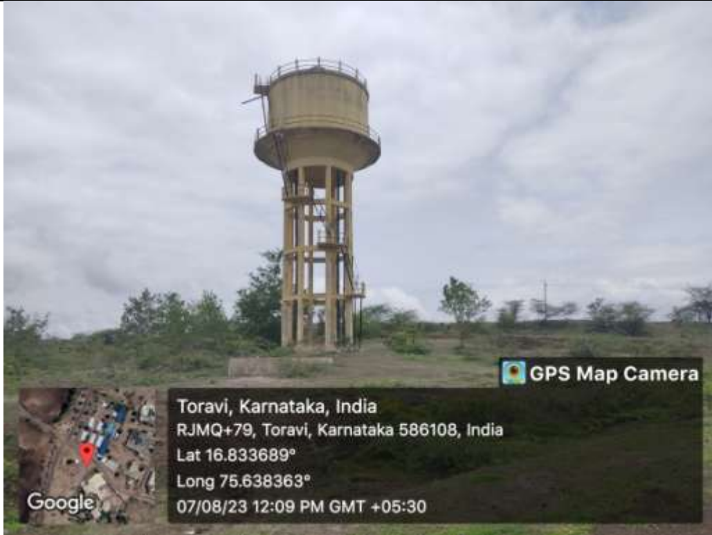
Water Storage Tank 2: ( Storage Capacity- 2.5 Lakh Liters)
