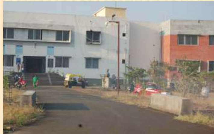
Asphalting road along with the cross drainage work near Social Science Block
